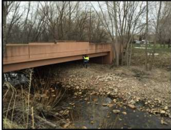
Deposition of Sediment at 41 st Street Bridge deposited in 2013 flood.
