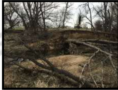
Tree fall on Boulder County Open Space from erosion spanning \frac{3}{4} to full channel width on Lefthand Creek West of Longmont
